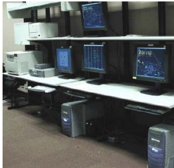
Figure 3. “Back room” installation of multi-center TMA at New York Center
